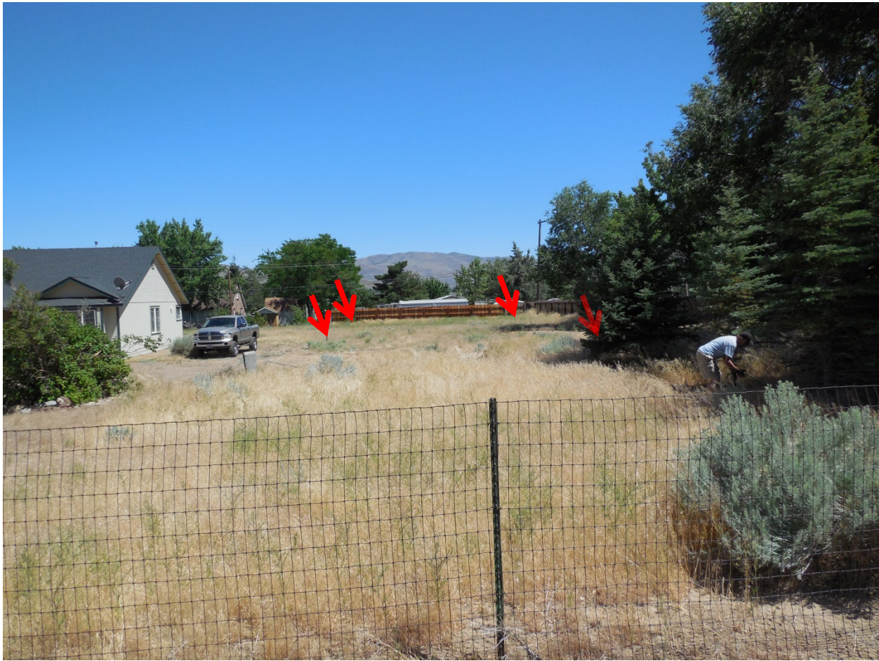
Corner stakes of building. The stake on the right is behind the pine tree
